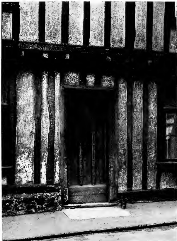
DETAIL OF DOORWAY HOUSE AT WYMONDHAM The vermicular design in the stucco is interesting
